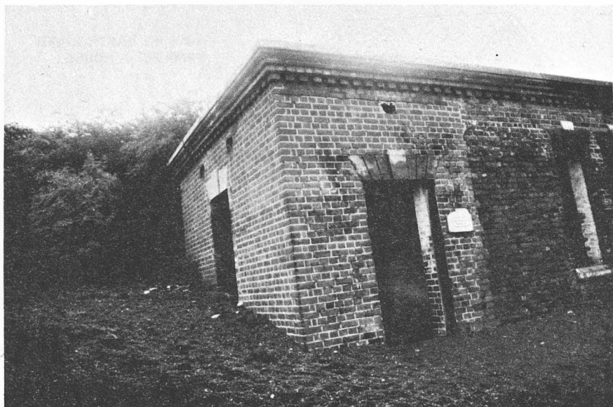
Subsidence caused by liquefaction (Kingston, Jamaica).
