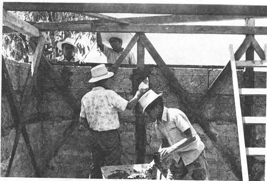
Local builders participate in building a safe house to learn better building techniques. (Photo: Mary McKay/World Neighbors)
