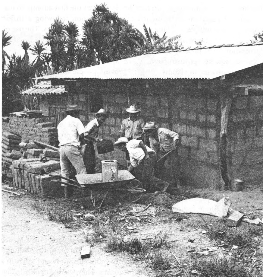
A Kuchuba'l Group works together to rebuild a house in a disaster area. (Photo: World Neighbors)
